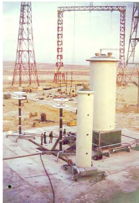
Outdoor impulse generator & multiple chopping gap 2400 kV
